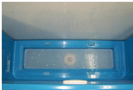
Figure 2: Showing the filter compartment with only the bottom grate installed.
